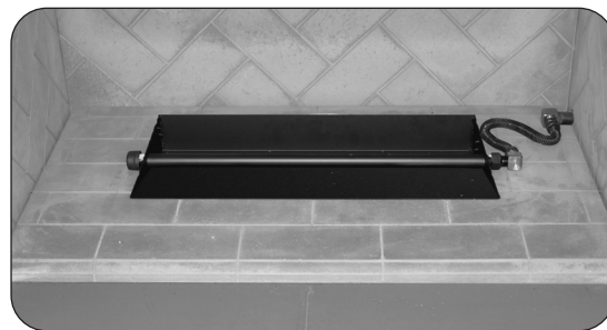
Fig. 10-2 Center burner in fireplace
