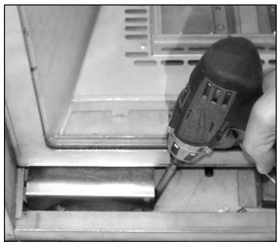
Power Vent Control Module Mounted inside fireplace.
